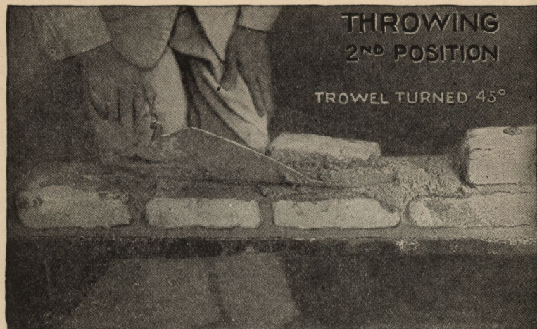
FIG. 3,965.—Throwing mortar—2 nd position. The trowel is gradually moved along the brick and turned at the same time—the point of the trowel rides along the center of the brick course without touching it.
