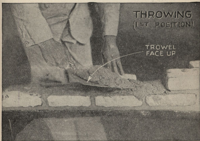
FIG. 3,964.—Throwing mortar— 1st position . Note trowel is being turned as it is moved along the brick.
