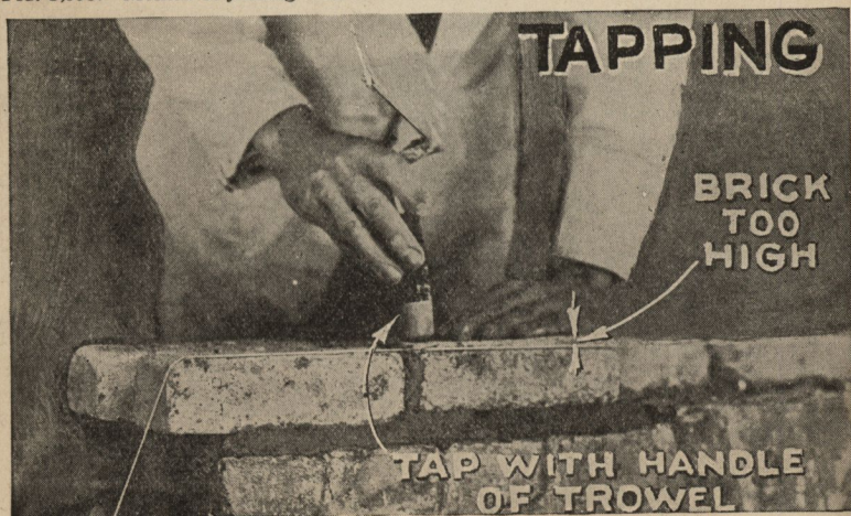
FIG. 3,996.—Tapping, or knocking down brick to level of lime, where brick is high because of excess mortar. A first-class brick layer will rarely resort to tapping. It is sometimes done though ill-advisedly, through force of habit.
