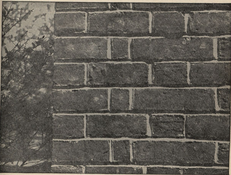
FIG. 4,105.—Appearance of concave joint Flemish bond, closers at corner. Concave and V joints are comparatively inexpensive to form and are weather resistive.
