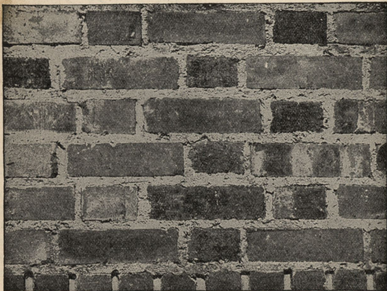
FIG. 4,104.—Appearance of flush joint Flemish bond. It is almost always finished with a rough texture. When used with rough texture brick it is difficult to keep the mortar from the face of the brick. Formed by cutting off mortar squeezed beyond the face of the wall. The joint
