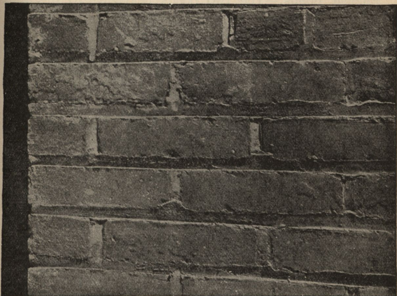
FIG. 4,091.—Appearance of struck joint common or stretcher bond. The mortar joint constitutes a considerable proportion of the area of the finished wall and hence should be considered as to its width, color, texture and section. With a standard brick, two headers require a \frac{1}{2} in. joint to coincide with the length of a stretcher. In forming bonds and patterns the \frac{1}{2} in. joint is thus most practical. Joints \frac{5}{8} and \frac{3}{4} in. wide are used extensively and are very effective, the difference between the unit length of a stretcher and two headers plus a joint being taken up by slightly varying the width of the vertical joints. Joints 1 in. and even wider have been used. A joint of \frac{3}{4} in. and over slows down the work, a thick bed of soft mortar under each brick being more difficult to manipulate. Special mortar should be used for wide joints.
