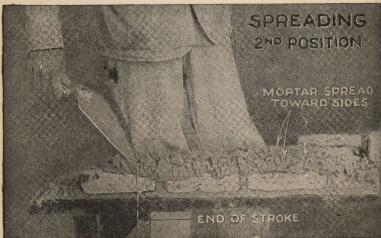
FIG. 3,979.—Spreading mortar— 2nd position . End of stroke. Note mortar spread out toward the sides of the brick hollow in center keeping mortar flush with sides, also note position of trowel at a small angle (about 45^\circ ) with face of brick.
