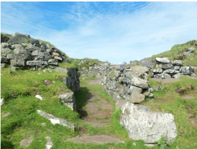
The walls of the broch show how carefully the builders used dry-stone-wall techniques to piece together very sound walls without the use of any mortar. It all depended on picking the right size pieces to fit together like a giant jigsaw puzzle.
