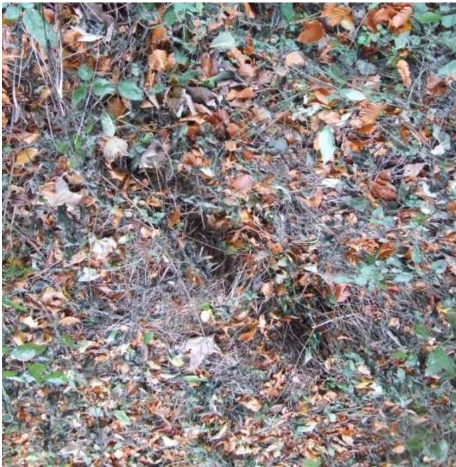
Hole in the ground outside the east wall of St Medden's church.
